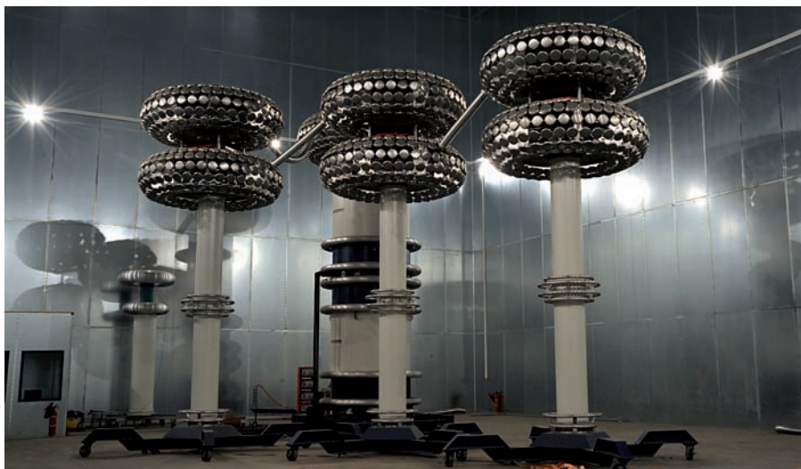
Shielded room for testing of EHV cables (France)
