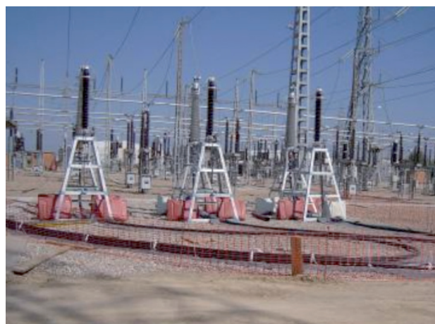
Typical use of stand-by link for maintenance in substations
