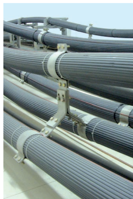
Cables installed in tunnel
